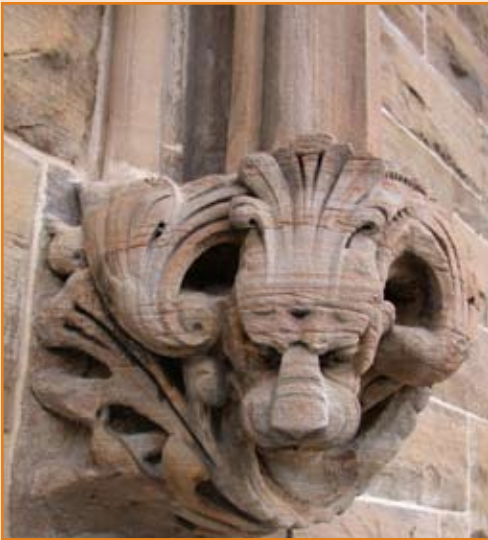
A decorative stone gargoyle after church restoration. Photo courtesy of Page Ayres Cowley Architects, LLC.
